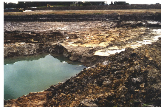
Exposed acid sulphate soil
